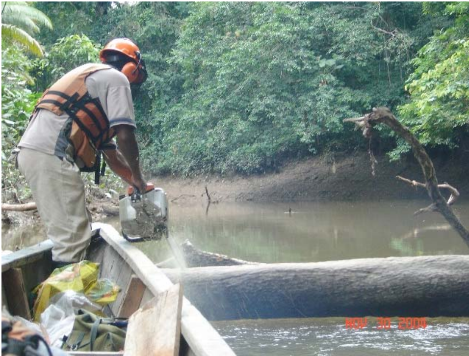
Fig. 10 – Opening a river for logistical access, this is difficult to restore and impacts areas upstream
